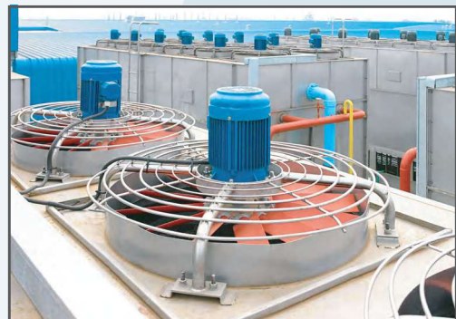
Fan and water pump
